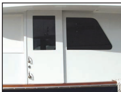
Installed side view, Closed window alignment
