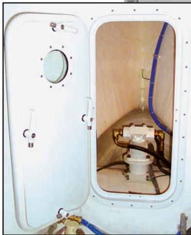
7" view port, Access to bow thruster
